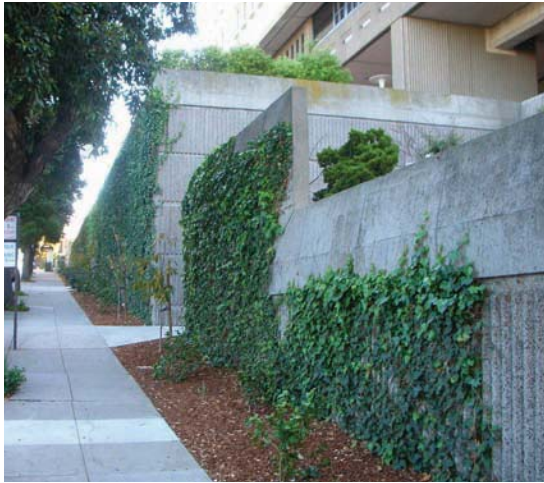
The entire street wall on the southside of Post Street between Laguna and Gough is comprised of concrete walls.
